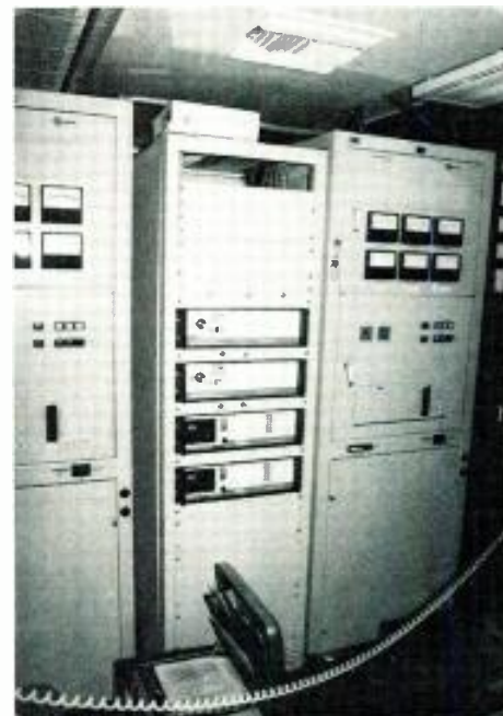
Control area of the truck where transmit/receive functions are executed.
